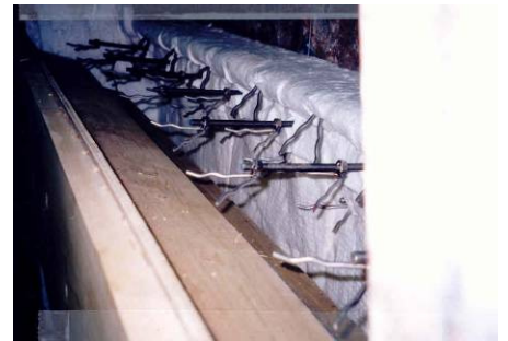
Custom anchors to retain shelf pour - 21" overall thickness (eliminates several tile pieces - lengthily delivery)
