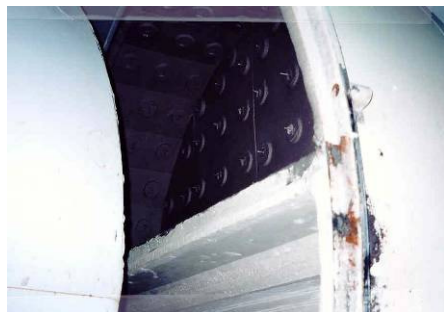
Use of 1/2" board as bearing ring prior to fiberlock washer. Surface coated with ITC-100 Ceramic Spray. Everything looks great.
