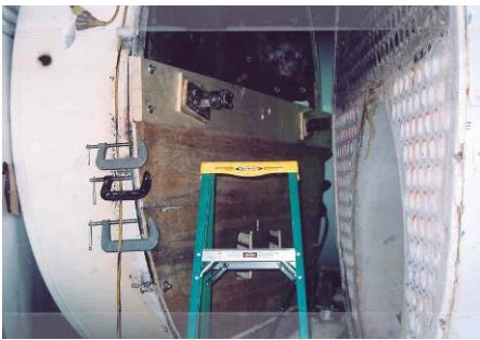
Lower door poured - approx. 65 units of Thermbond Formula Nine (shelf area used stainless fibre addition).
