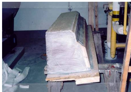
Shelf portion of the lower door coated with lithium grease.
