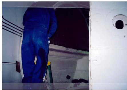
Lining of the upper door section 2", 8# blanket, followed by 1/2" vacuum formed board.
