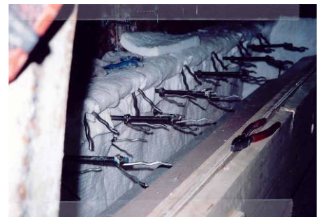
Backup insulation 8# density ceramic fibre covering I beam in the centre of the door.
