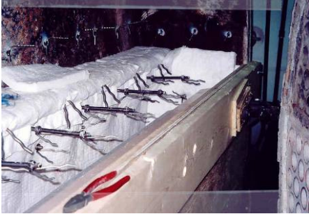
Upper door using fibre lock anchors to retain 2" of 8# density blanket and 1/2" thickness of vacuum formed board.
