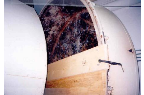
Shelf portion of the form in place after lower section has been cast.
