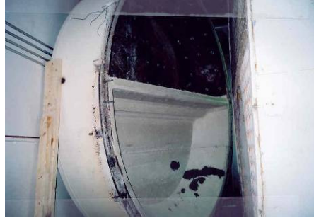
Wesmat uses vibrators mounted on the form and operates them throughout the pour.
